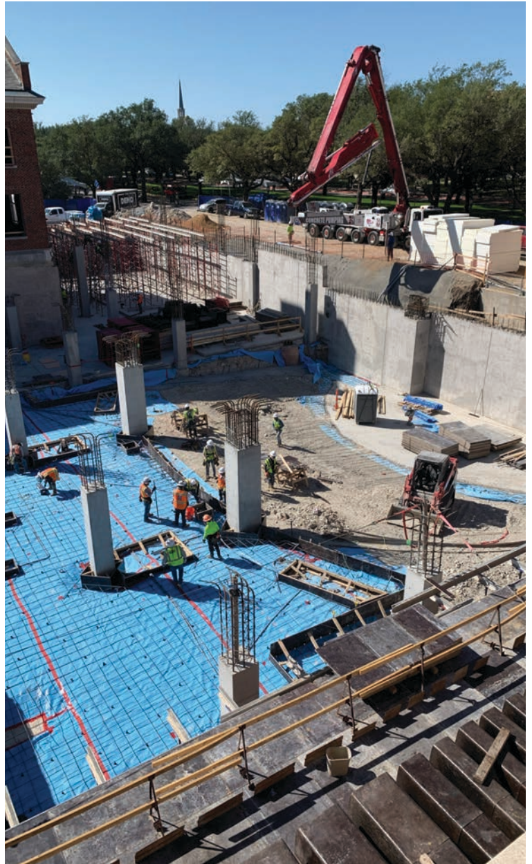
By October, all evidence of the old Business Library and the exterior steps had been removed. This photo was taken from the front of the Maguire Building looking toward Bishop Boulevard.
