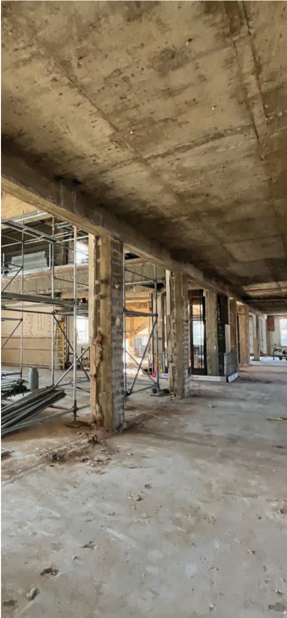
Down to the studs in the Fincher Building hallway. This is the view just outside the EY Gallery.
