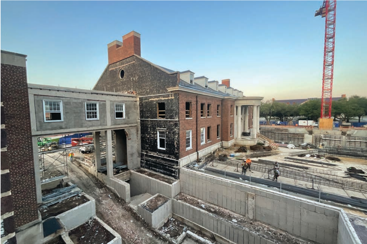
The “bridge” that connected the Fincher Building to the Crow Building, and the columns and stairs beneath, are on the way to being demolished in this photo, taken mid-summer.
