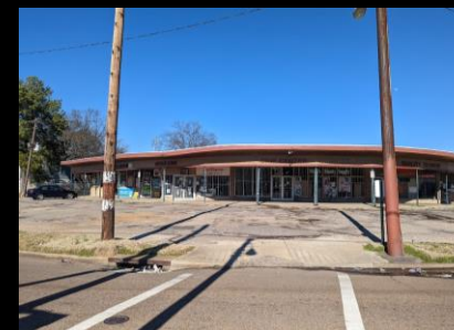
Dilapidated commercial building
