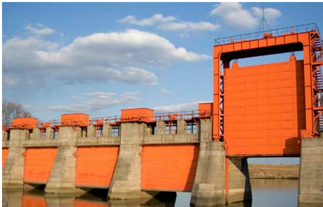
Example of Flood Gate
