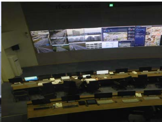
Fig.5: Songdo Control Room, Sept.2,2013
