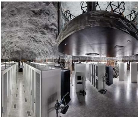
Fig.8 Pionen Datacenter, Stockholm Sweden
