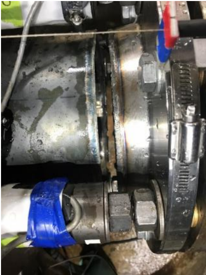
Figure 3.4. TTS north end cap failure
