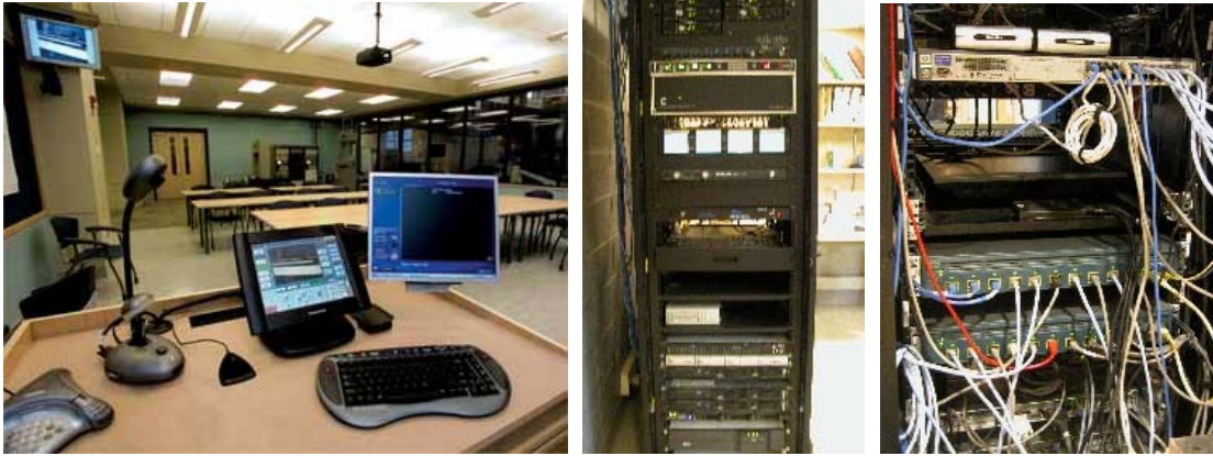
Figure 1. Views of the Electronic Conference Room and Equipment
