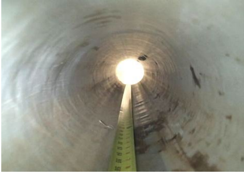
Photo 4. Image of Specimen 3 Liner after First Rotation Testing Showing No Crack
