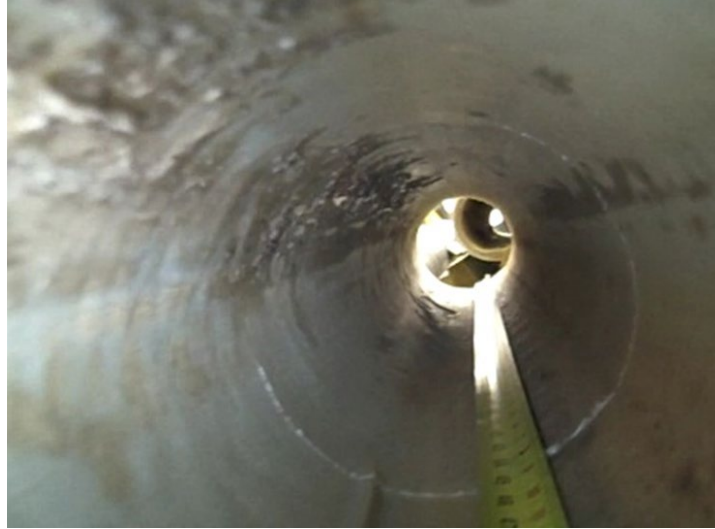
Photo 2. Image of Specimen 1 Liner after First Rotation Testing Showing a Crack at the Center
