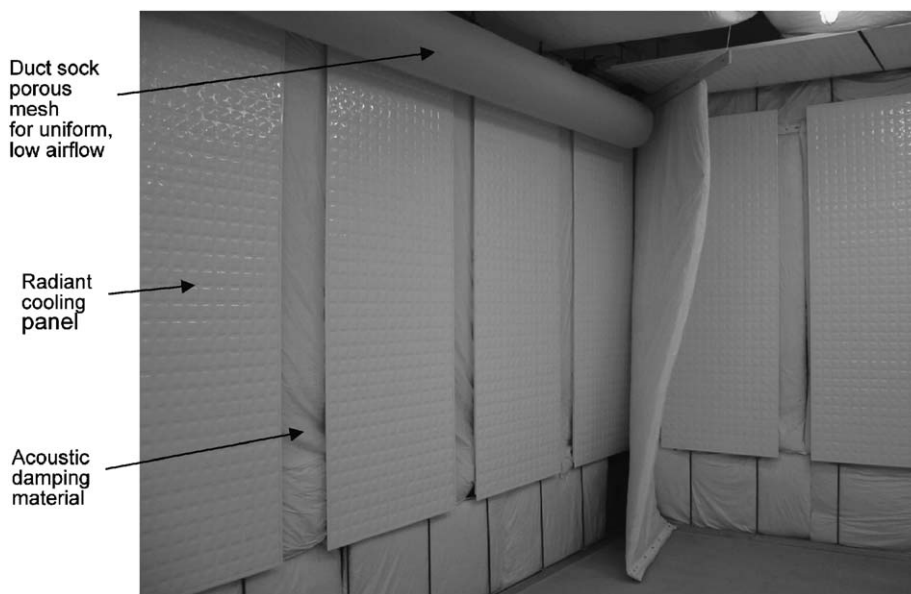
Fig. 5. Photograph of the STEM room at Bell Labs circa 2002. Fiberglass acoustic banners are hung \sim 6 in off the wall and behind the radiant cooling panels. When filled with water, the cooling panels are rather poor sound reflectors. The air supply to the room is connected to a duct sock which diffuses air along its entire length, rather than in drafts as with vented supplies.
