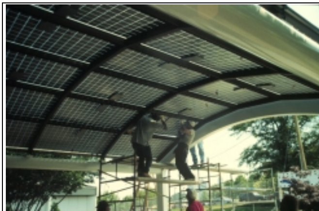
Fig. 2: A semi-transparent Solarex BIPV array serves as the entry canopy of the natatorium at the Georgia Institute of Technology in Atlanta, site of the 1996 Summer Olympic games. The building also features 350 kWp of roof-top BIPV. (Solar Design Associates, Inc.)
