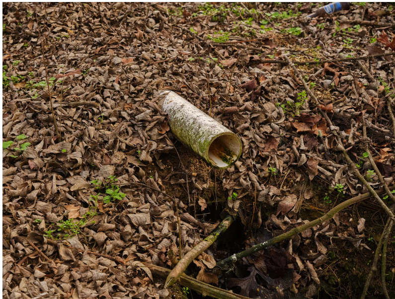
A PVC pipe behind Ms. Rudolph’s house spews raw wastewater whenever someone flushes the toilet or runs the washing machine. Matthew Odom for The New York Times
