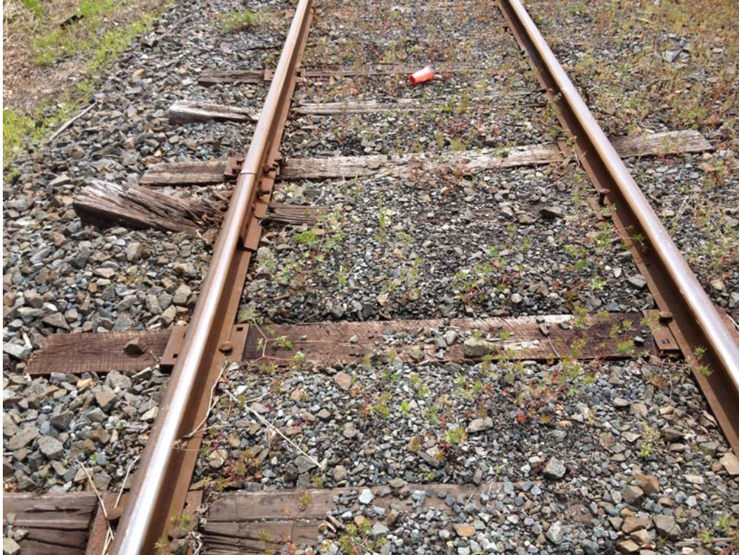
Figure 9: Poor tie conditions
