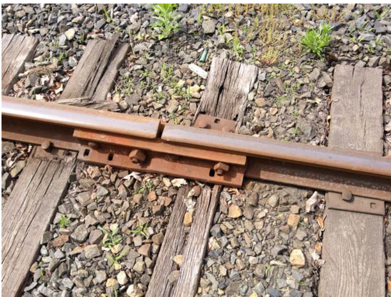
Figure 6: Compromise Joint Bar Between two different rail sections
