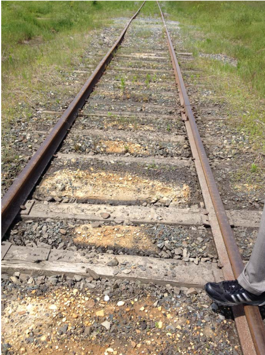
Figure 7: Surface degradation on 85 lb. rail track
