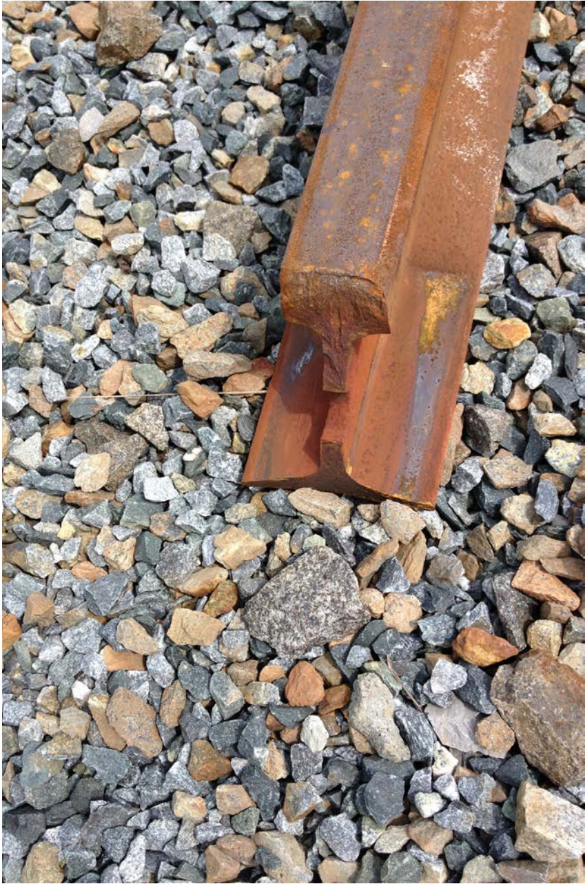
Figure 4: Bolt Hole failure
