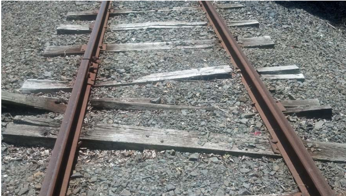
Figure 12: Significant Tie Movement Due to Running of Unanchored Rails
