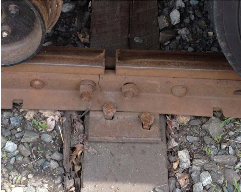
Figure 5 Broken Joint Bar
