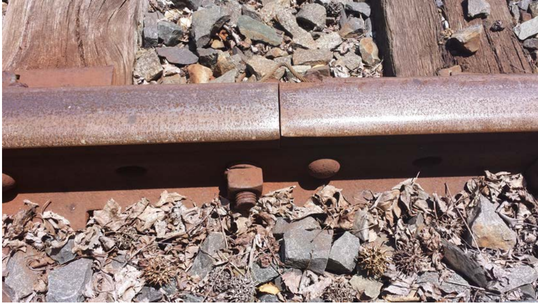
Figure 11: Observed Tight Joints
