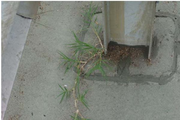
Figure 4. Bermudagrass growing around guardrail beam where caulk malfunctioned.
