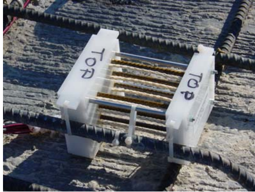
Figure 5 Corrosion penetration monitoring with CPMP
