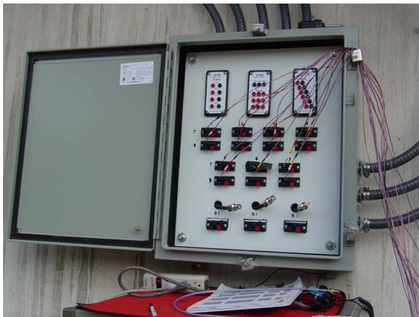
Figure 5.2 Set Up of the Junction Box
