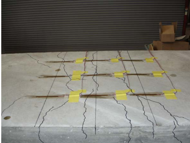
Figure 4.27 Continued Cracking throughout the Interior Pier Concrete Slab Region during Deflection Steps 5 through 8
