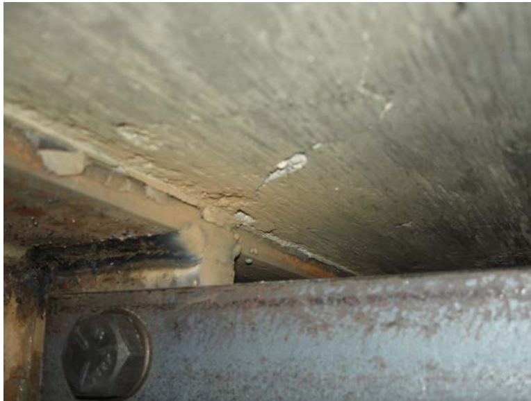
Figure 4.30 Large Crack on the Bottom of the Concrete Slab at the East Actuator as Revealed after Experimental Testing
