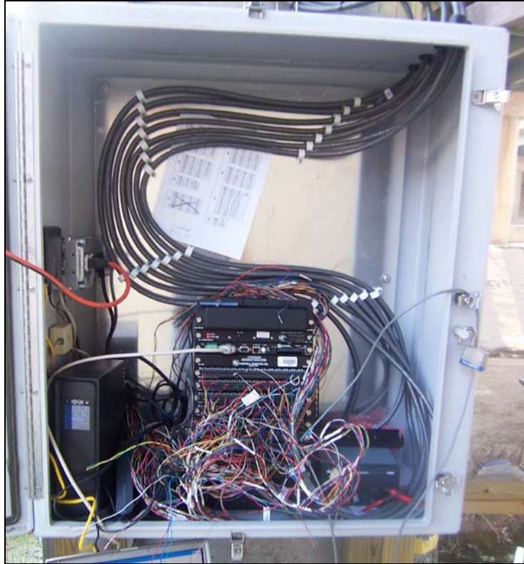
Figure D.1 Interior of main fiberglass box
