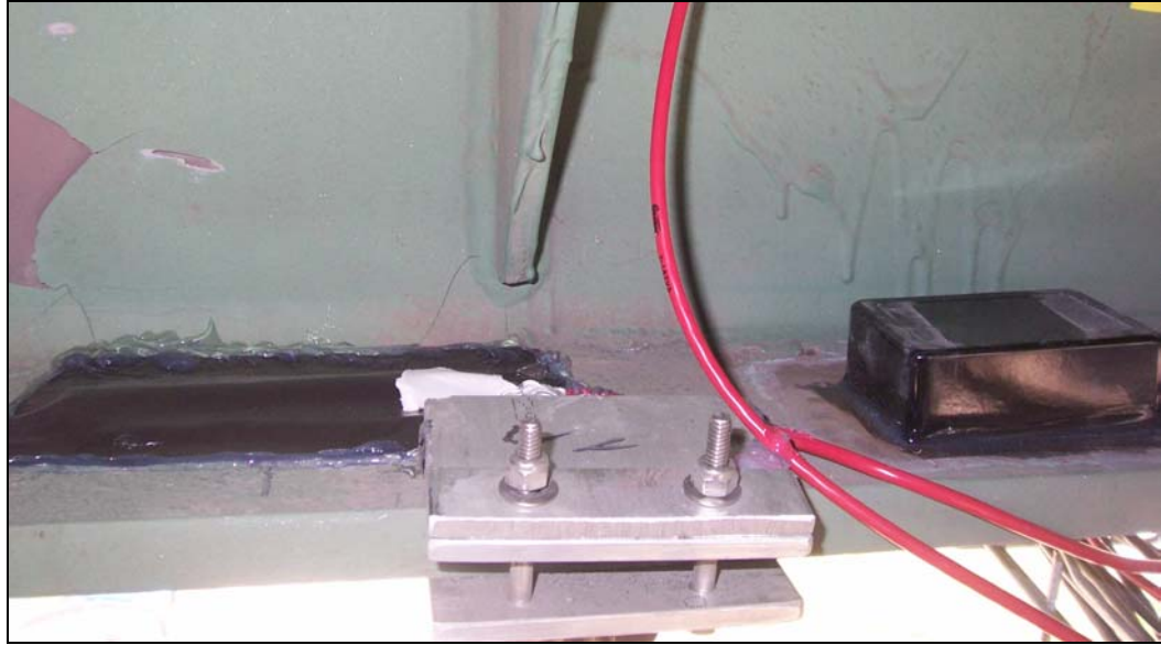
Figure D.8 Enclosed vibrating wire and foil strain gages
