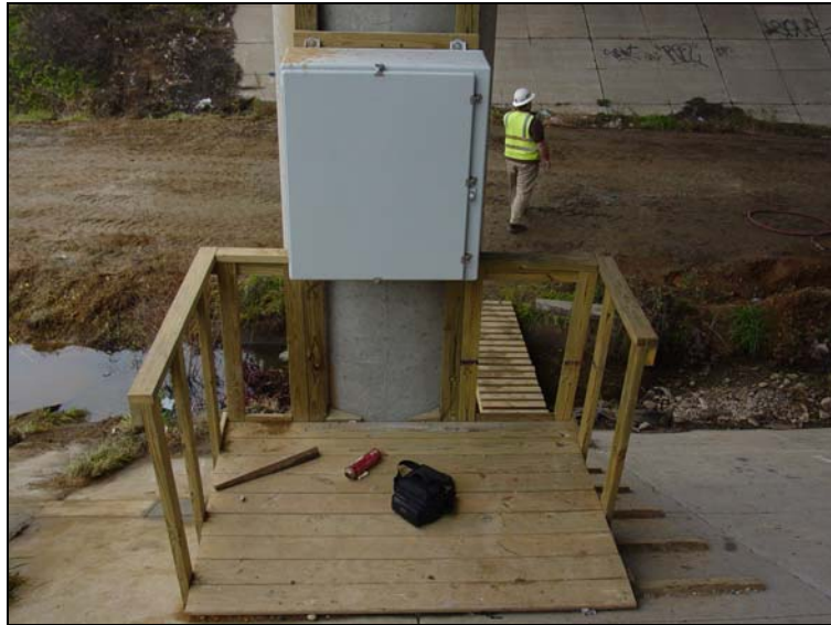
Figure 6.15 Photo of platform & fiberglass enclosure
