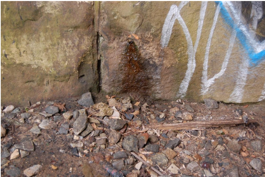
Figure 8.9. Photograph of Port 5 in September 2011. The leachate appears clear and there is no evidence of significant iron oxide precipitate on the gravel or abutment wall.
