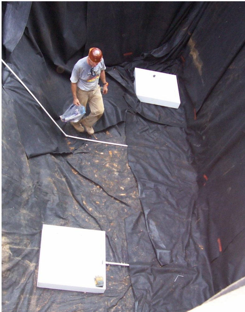
Figure 8.2. Photograph of two of the three leachate basins installed at the bottom of the South Embankment.
