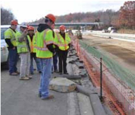
Sam Bostick leads students on a tour of the Newark, DE High Speed Toll Facility construction site.
