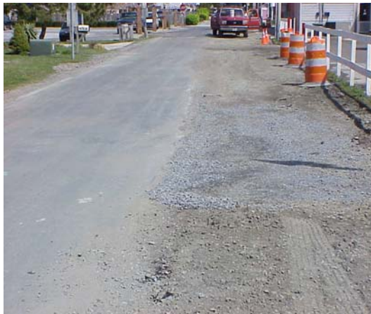
Significant portion of this road was damaged by a utility trench
