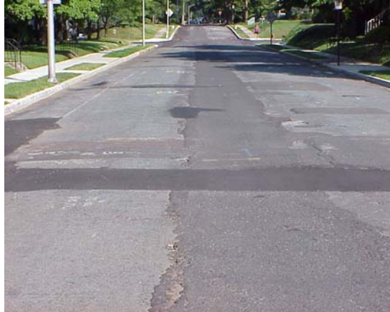
Road destroyed by Utility Trenches
