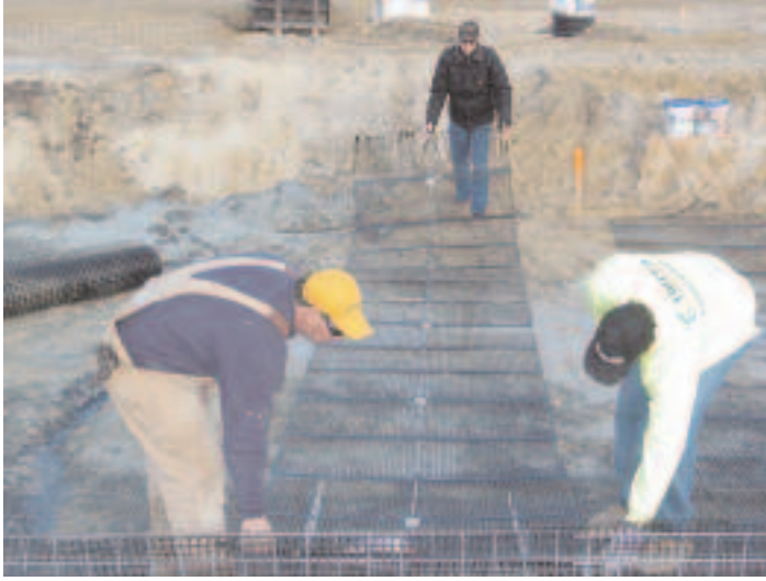
The research team works on installation of the MSE wall monitoring system. Five strain gages are attached to each layer of 22-ft-long geogrid. The surface is abraded and heated, and the gages are then attached using epoxy. The layers are spaced vertically at 1.5 feet, and every other layer is instrumented.
