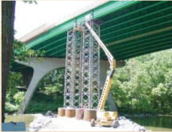
Temporary jacking towers are installed to enable the bridge to be repaired with steel plates.
