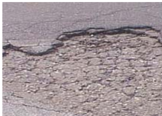
Overlay failed because the underlying failure was not addressed
