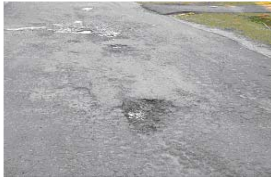
Failure of asphalt binder course prior to placing the final wearing course
