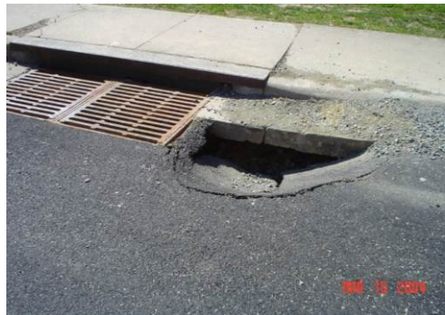
Pavement failure at storm inlet due to poor backfill practices
