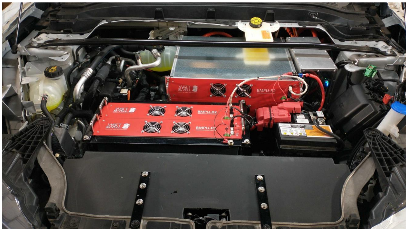
Figure 3.1. Photograph of the four Watt & Well BMPU-R2 converters (bidirectional chargers) installed in the front “frunk” of a Ford Mach-E. The converters are recognized by their red front panel, each with two cooling fans. To the right of the rightmost converters is a UD junction box with power connections and UD’s logic board to run LIN-CP and CAN communications.
