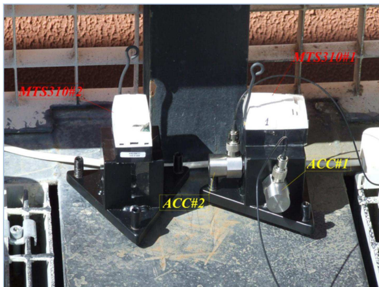
Fig.5 – Detail of the sensors layout on the bridge axis
