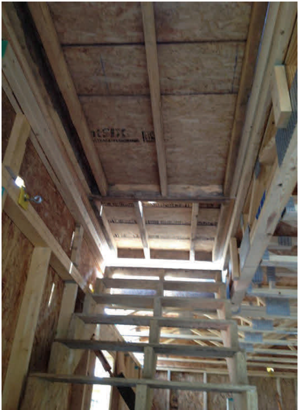
Figure 10: Stair Opening Covers from Lower Level
