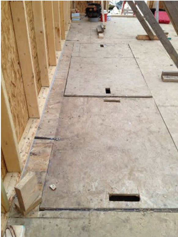
Figure 9: Stair Opening Covers Sections
