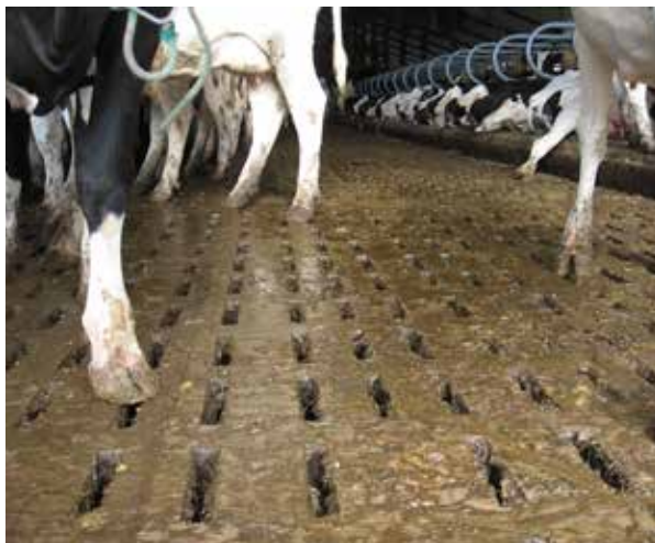
Figure 8.12 Slotted floors, like this example in a dairy barn, cover a manure storage that may be up to 10 feet deep, usually referred to as a deep-pit storage. Slotted floors are also used extensively in swine facilities. Credit: PSU Ag Safety.
