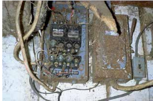
Figure 5.42 Improper electrical wiring methods and materials placed in a hostile farm environment can lead to fires and electrocution of people and livestock. Credit: PSU Ag Safety.
