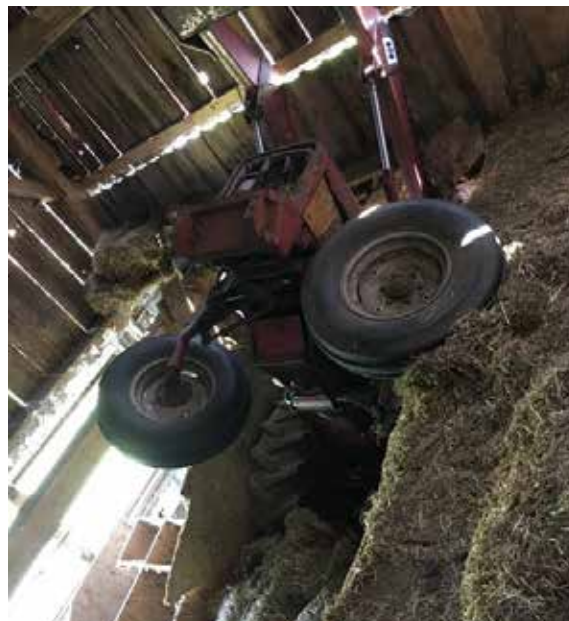
Figure 0.3 The old wooden floor gave out beneath this tractor in a 19th-century barn. Credit: Joy Drohan.
