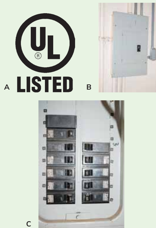
Figure 5.41 Electrical components are built to strict safety standards and tested for reliability by the Underwriters Laboratory (UL). Look for the UL label (a) to help ensure the safety of electrical equipment. You may have to operate circuit breaker boxes (b, c) as switches for electrical tools. If the appliance suddenly stops working, then a GFCI, circuit breaker, or fuse may have broken the circuit to protect you and the wiring. Credit 5-41a: UL, LLC Credit 5-41b, c, d: J. Mathison.
