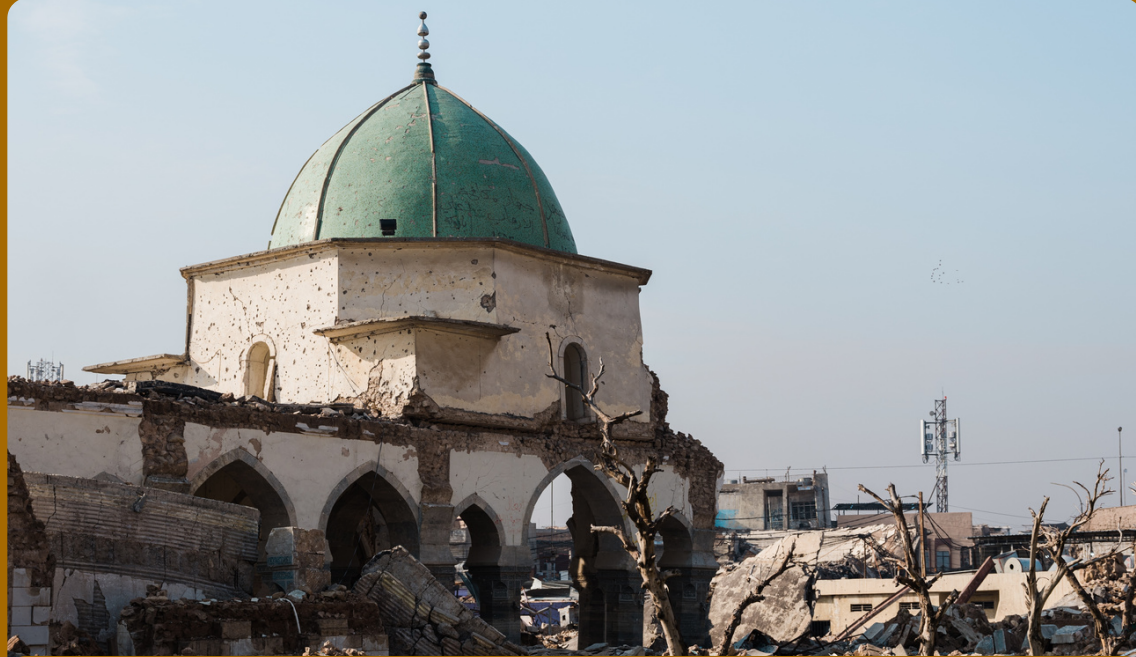
The central dome of Mosul's Great Mosque of al-Nuri following an explosion by the IS in 2017 (Chris Pook/Shutterstock, November 2018)
