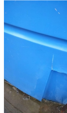
The cracked water tank in Cebadilla
