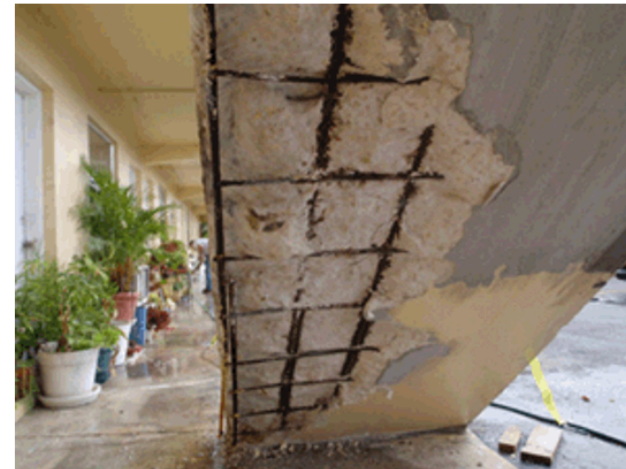
A typical case of corrosion in reinforced concrete
