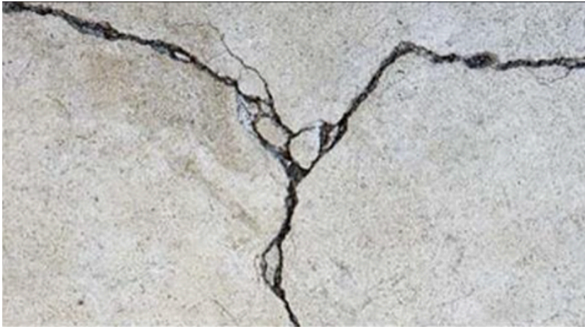
Crack in concrete
