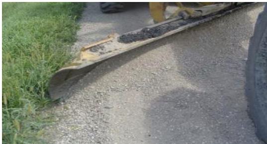
Figure 7. Blading being performed on an unpaved road. The moldboard is used to drag loose sediment across the road surface.
