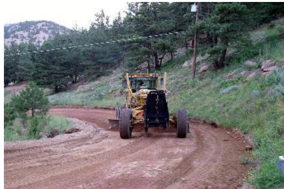
Figure 8. Grading being performed on an unpaved road. The road grader (tractor) cuts the surface of the road and refills the cut surface with aggregate materials.
