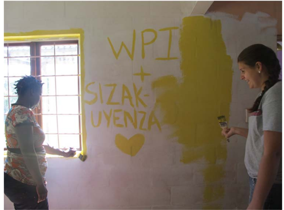
Figure 6: Collaboration was essential as we worked together to paint the interior of the Safe House.
