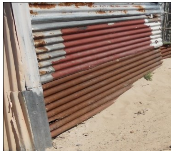
Figure 10: Sand piled along the base of a shack
