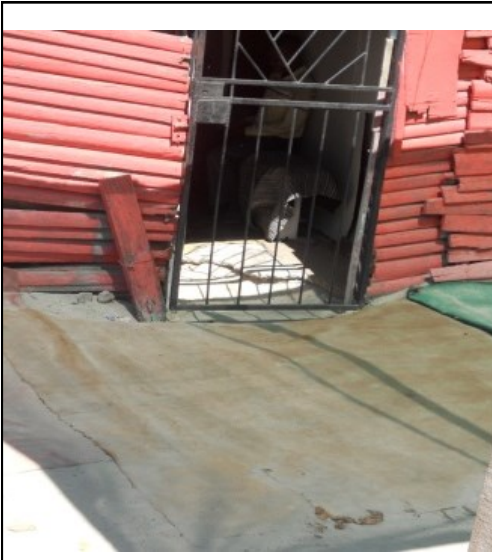
Figure 7: Shallow hole in front of a residence doorway
